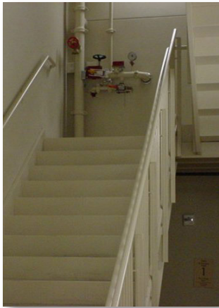
Fire protection system & fabricated metal stairs
